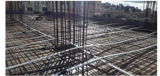
06 Ducts draped over a column line.
